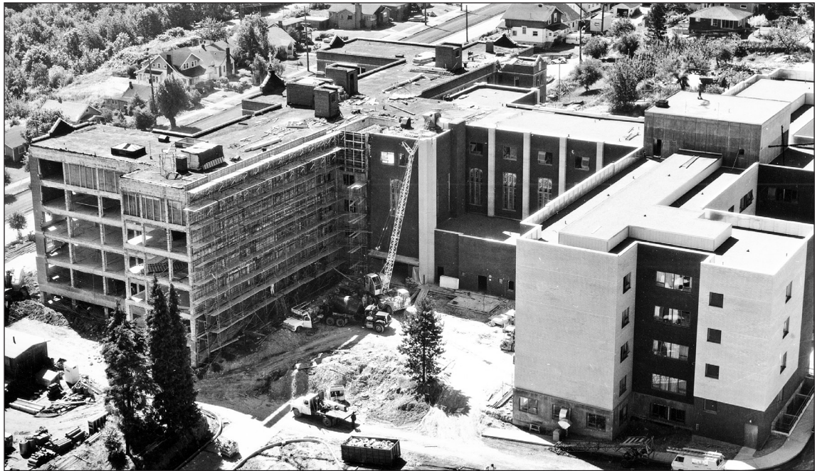
A closer view shows the transformation of the Mount, with the east wing (left) completely stripped of the old exterior and the west wing (right) faced with new brick. Note the chapel windows in center. Image #140.A3.11
